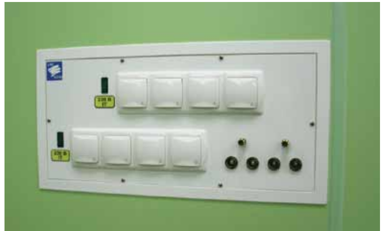
Built-in electrical supply console
