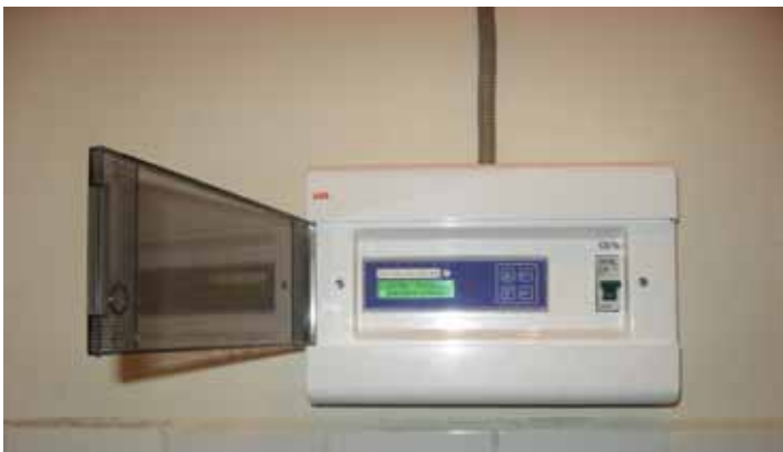
Medical gases control system
